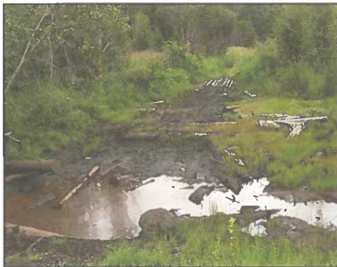
Above: A crossing of Leaf Creek, north of Nikiski. It is hard to imagine salmon trying to navigate through this mess. KWF replaced this crossing with a bridge in 2007.
