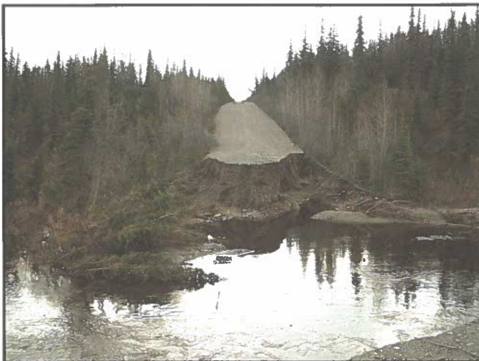
Above: This photograph was taken shortly after a road/culvert failure on Silver Salmon Creek. Access to several homes and recreational cabins in the Caribou Hills was cut off for several days before a temporary fix was installed. Shortly after, KWF replaced the culvert and restored the stream. This is a perfect example of what can happen when roads and stream crossings are build sub-standard.
