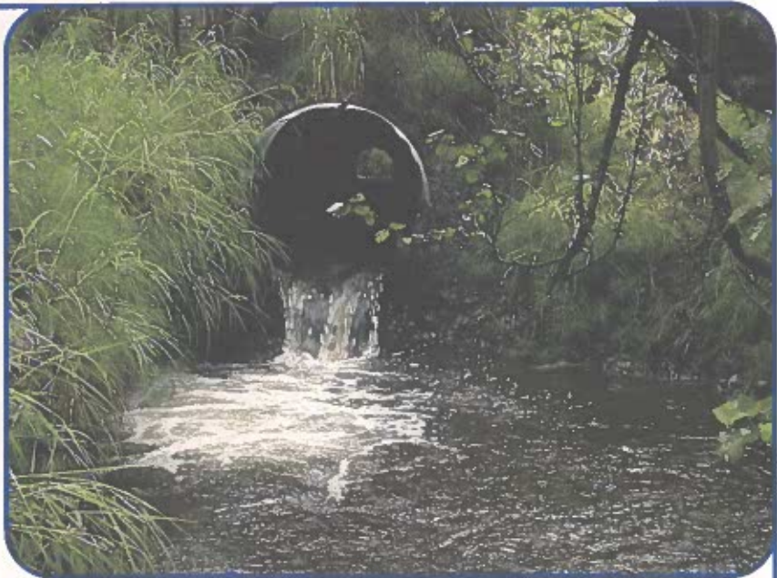
Raven Road crossing of Bean Creek: Culvert is "perched", meaning it is too high relative to the natural stream elevation. While evaluating this site, we witnessed an 8-10" fish leaping unsuccessfully to try to get upstream. This culvert blocks access to 1.3 miles of known upstream salmonid habitat.
