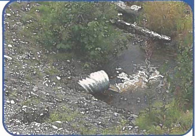
Above: "Perched" culvert at the Stariski Creek Pepper Road Crossing
