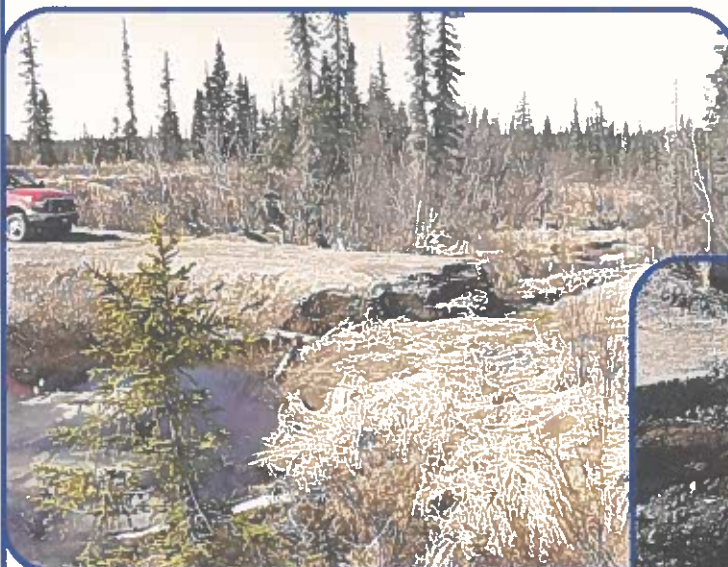
Above: Road washout.
