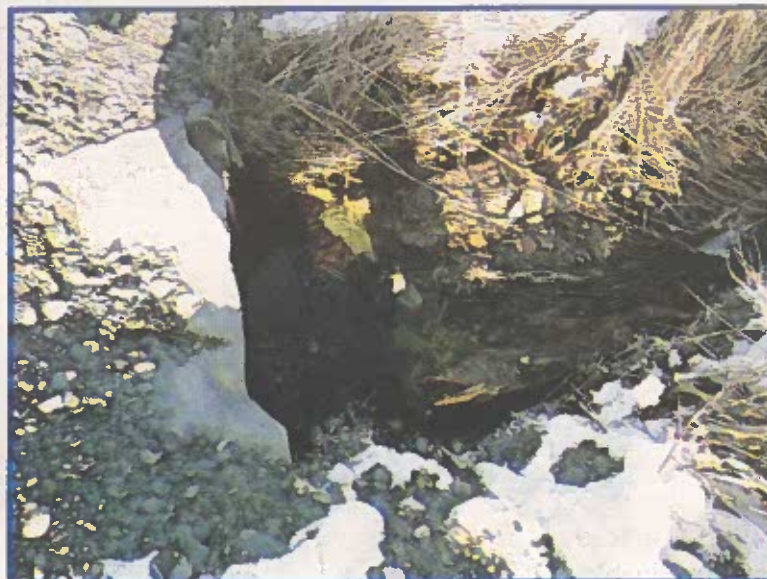
A crushed culvert impeding fish passage River Center Photo
