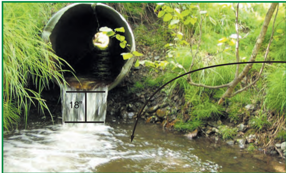
Culvert at Raven Road crossing of Bean Creek. This culvert was improperly sized and perched 18" above the stream. Juvenile fish cannot make this leap, so several miles of salmon habitat were blocked.
