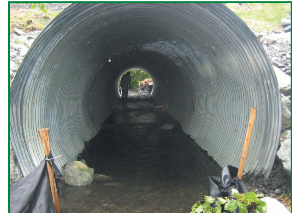
Success! Moments after water was released into the new culvert, we were able to stand on the bank upstream and watch juvenile king salmon jet through the new culvert.
