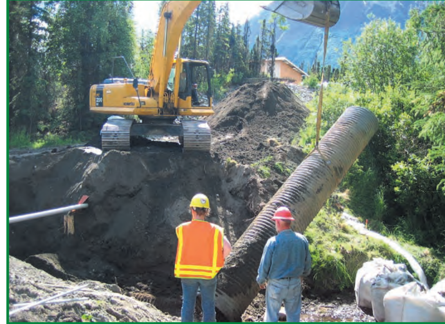
D&L Construction did an outstanding job on this project. Here they are removing the old pipe.
